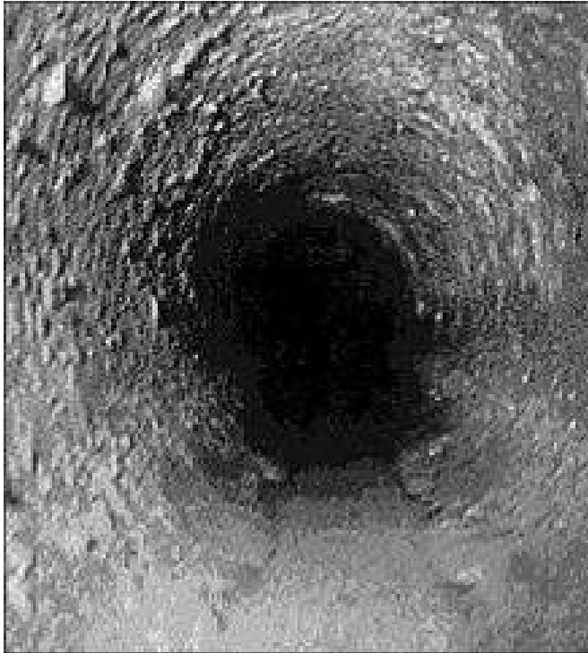
Pipe sediment build-up progressively constricts flow and reduces service
